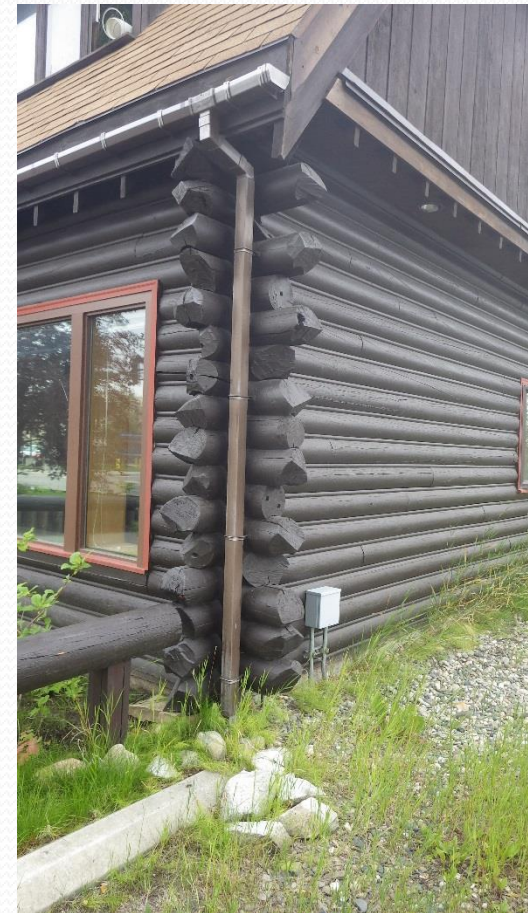
Drains that guide water to landscape
